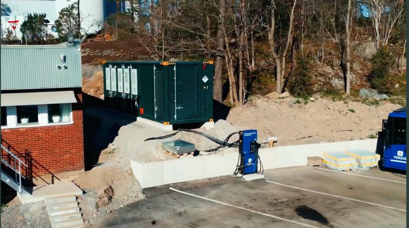
Sparq Supercharger deployed at Verdis, Stockholm, Sweden, in May 2026
