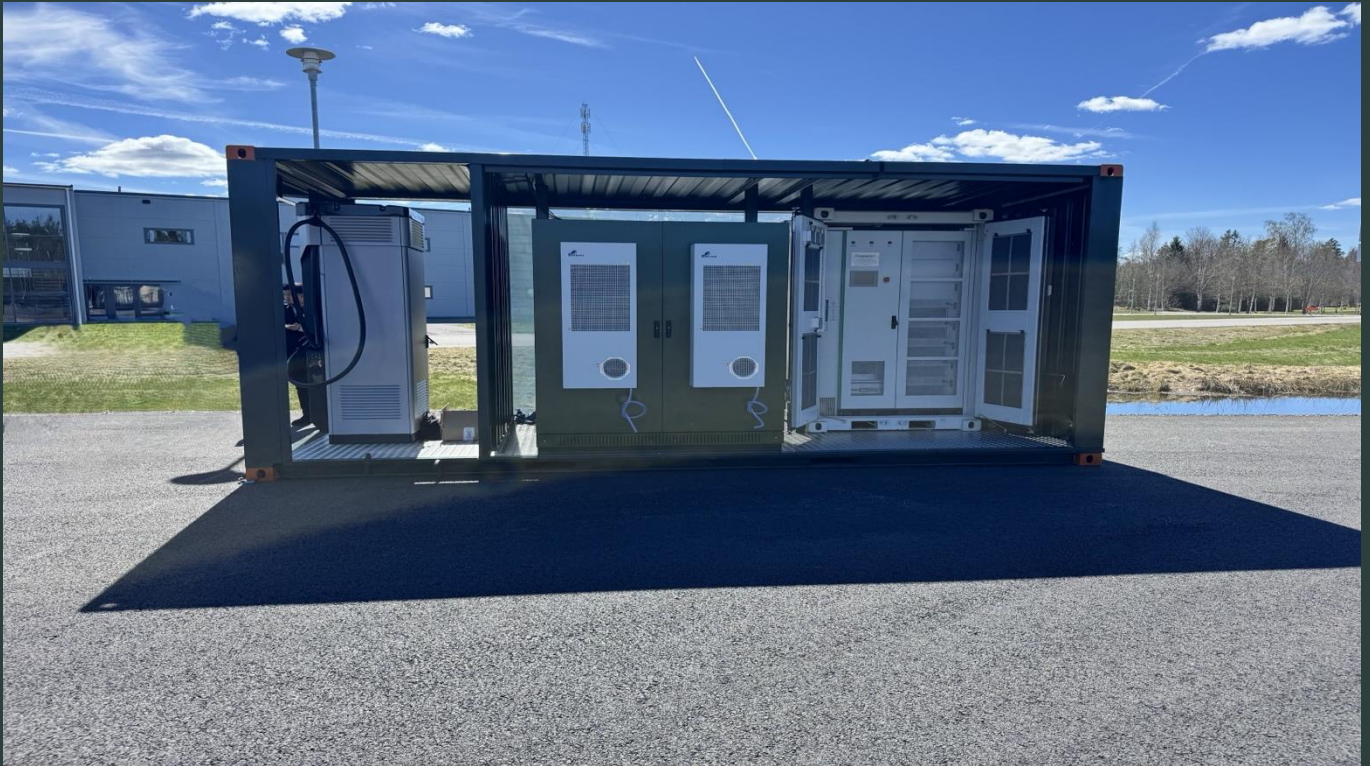
Sparq Mobile charge deployed in Älgult, Sweden, in April 2026
