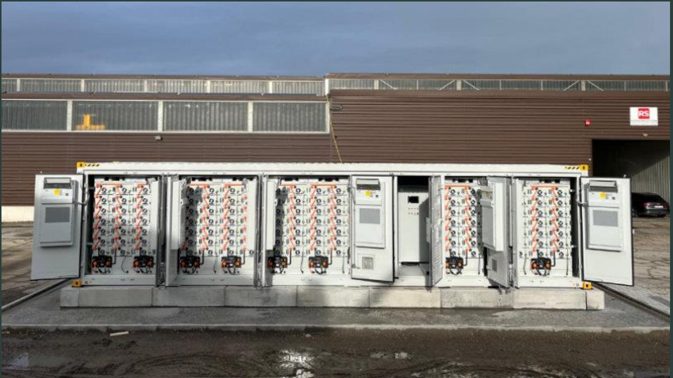
BESS deployed in Belgium in February 2026
